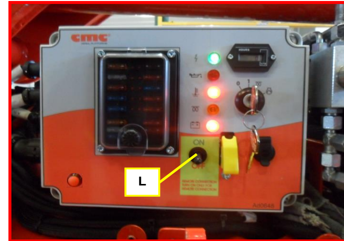
Picture 121: chassis box.
