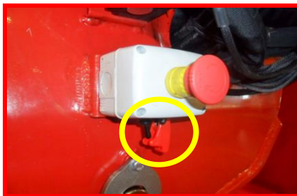
Picture 45: travel block bypass.
