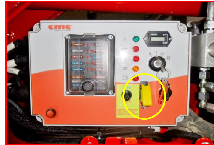
Picture 52: emergency bypass lever.
